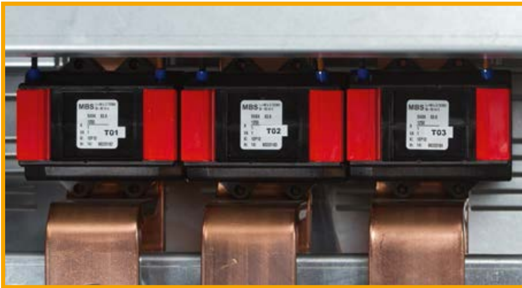
Fig. 9 Protection current transformer set
