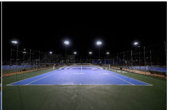
Bright, low-flicker illumination on the tennis courts
